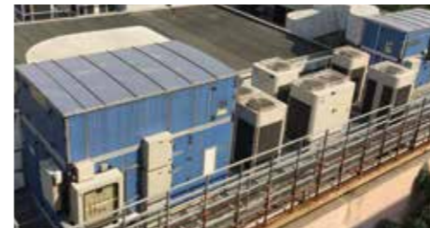
Cheung Ching Community Centre / Hong Kong - Installed in 2017
